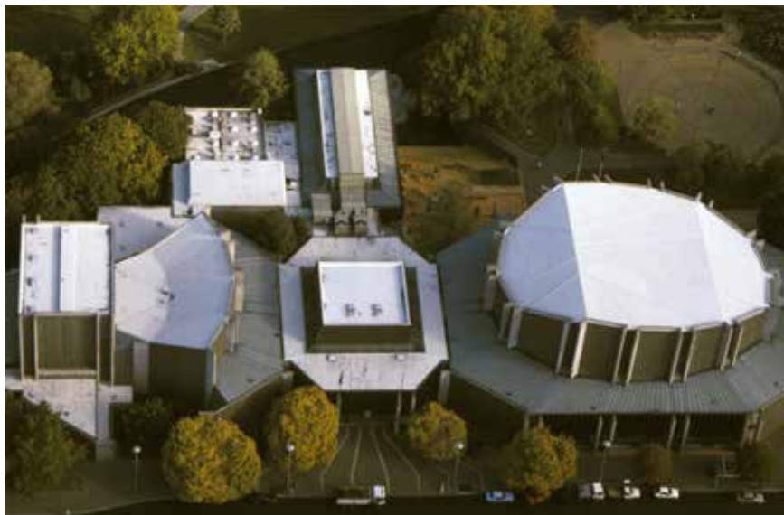
1mm Butynol laid in 1972. The main auditorium roof is still in service after 39 years. Some of the other low slope roofs are due to be upgraded with new Butynol during current building refurbishment.
